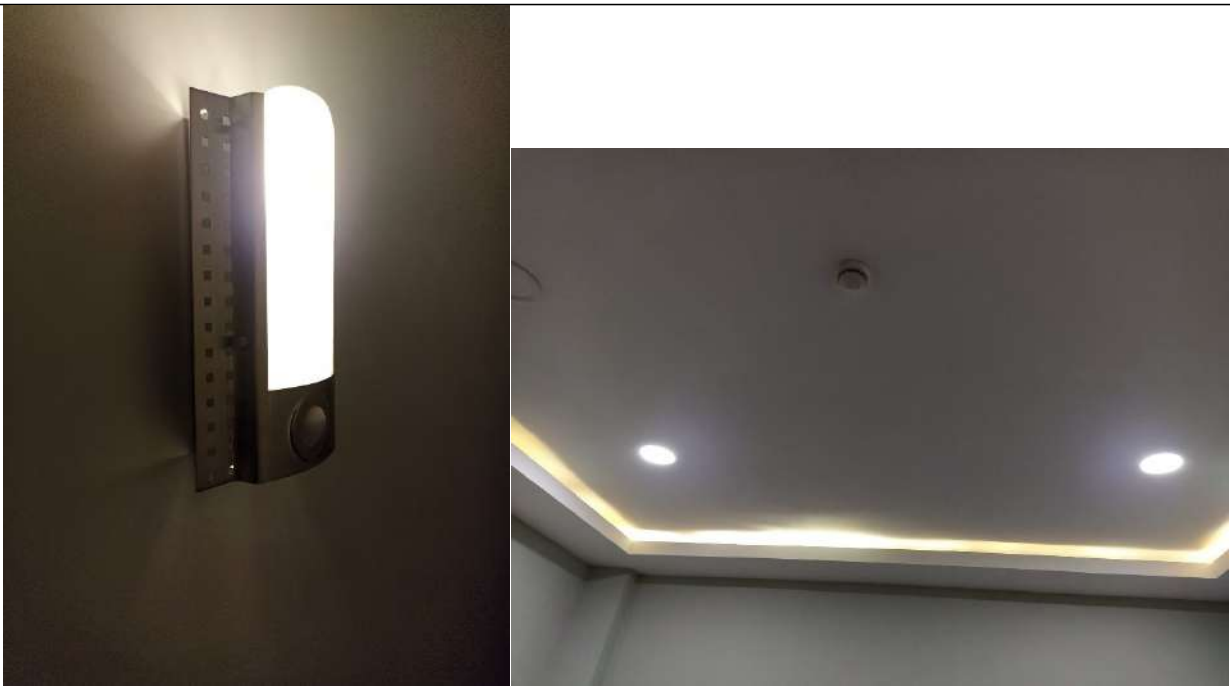
Example of Energy Efficient Appliances Usage: Use of LED lighting and lamps with light detection (Gaziantep University)
