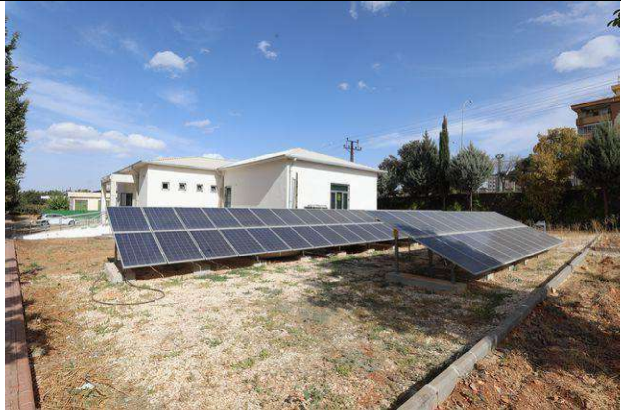
Energy House Management center Solar Energy Panels
